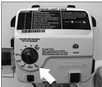
Figure 46 - Gas control valve.
